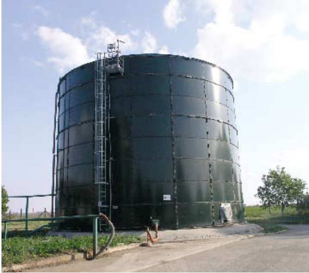
Storage facilities for slurry must be of appropriate capacity
